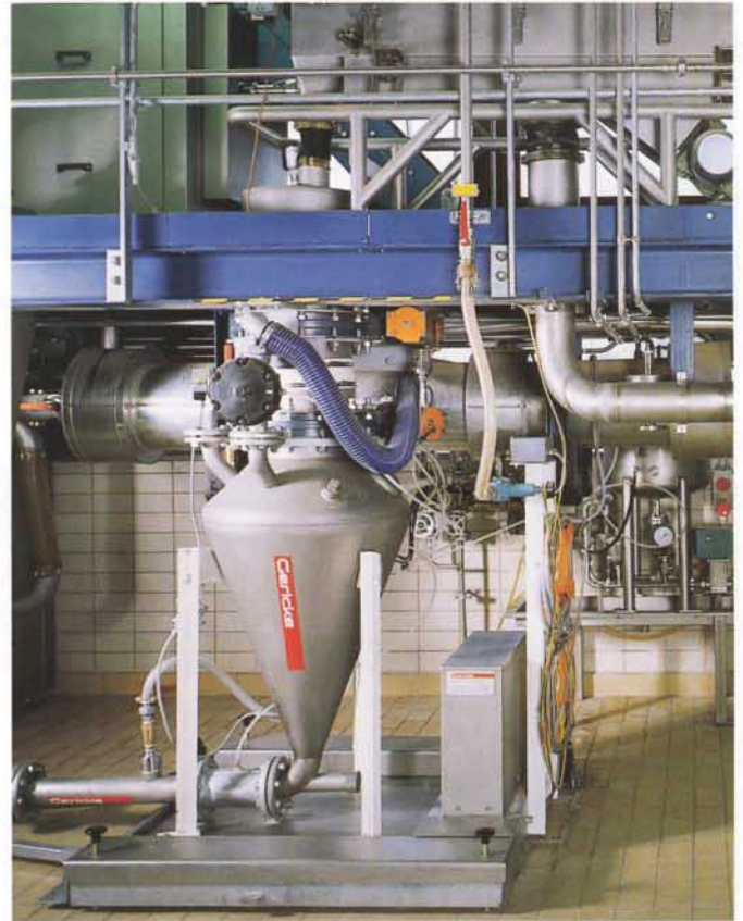
Pneumatic dense phase conveying
